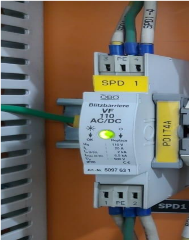
Fig. 11 Surge Protection Device Class D, 110 V AC
